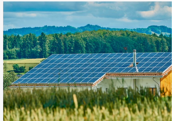
Photo: SolarX installation.
